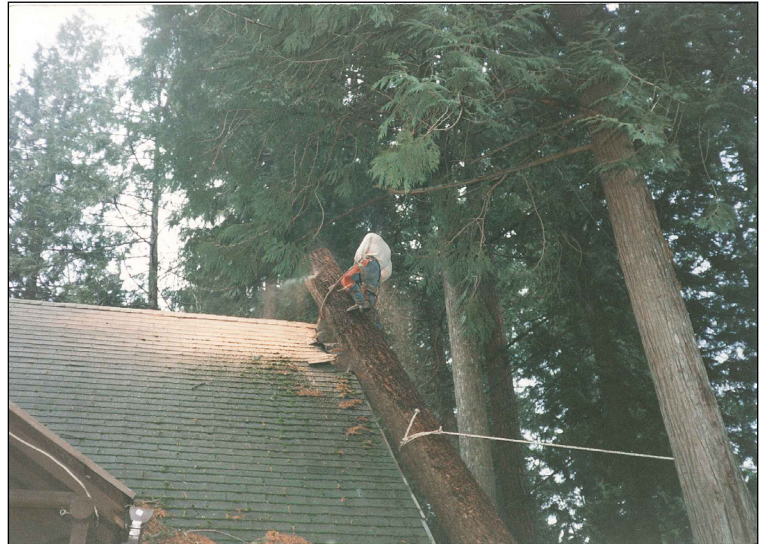
Three days after Coni and Terry purchased the property, a large Douglas-fir tree fell across the cabin roof, nearly separating the chimney from the house.
